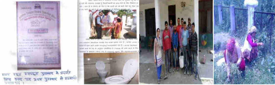
SMCs along with teachers providing their services to white wash/ clean school building /campus and preparing beds for kitchen garden:
